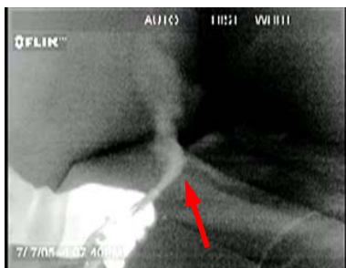
Figure 3A. Small amount of methane from nozzle.
