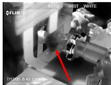
Figure 5c. Leak from LPG pumping station transfer line.
