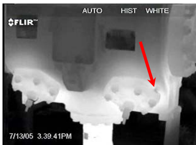
Figure 5b. Leak from LPG compressor right flange.
