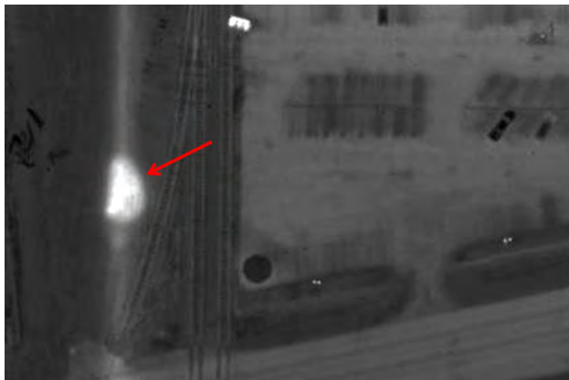
Figure 4a. Infrared image of a steam leak in a steam distribution line.
