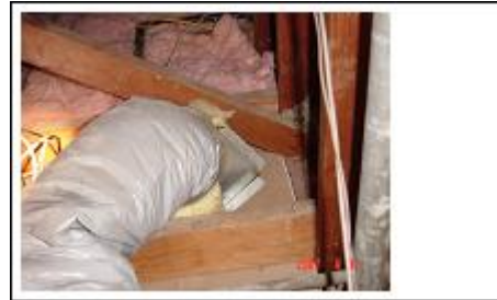
Figure 12b. Attic photo showing duct not installed and blowing air into attic
