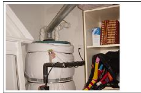
Figure 18b. Visual picture showing insulation pulled down at top which shows tank temperature vs. insulated temp.
